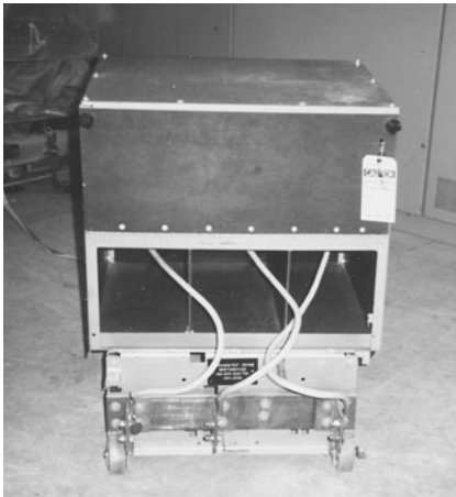
FIGURE 2.67 Front view of a 15-kV grounding switch. (Courtesy UNO-VEN Refinery, Lemont, IL.)
