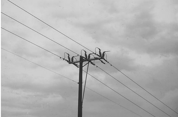
FIGURE 3.16 Mechanism-operated, three-phase, open-air switch. (Courtesy Alan Mark Franks.)
