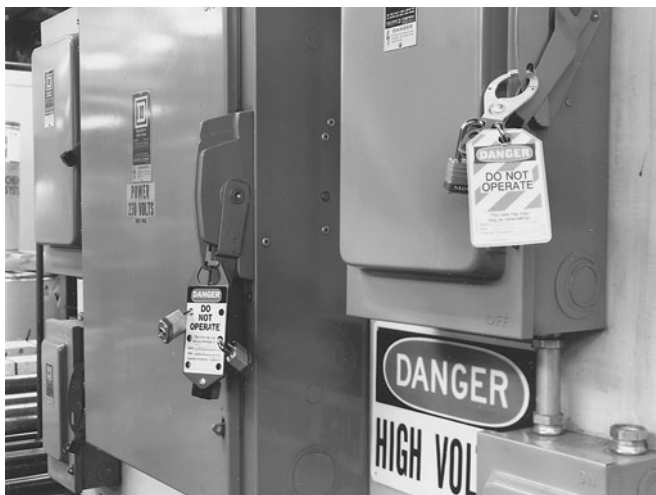
FIGURE 2.57 Typical application of locks, tags, and multiple-lock devices. (Courtesy Ideal Industries, Inc.)
